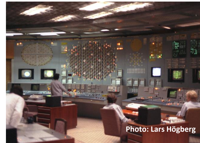
An RBMK control room (Ignalina 1990)
