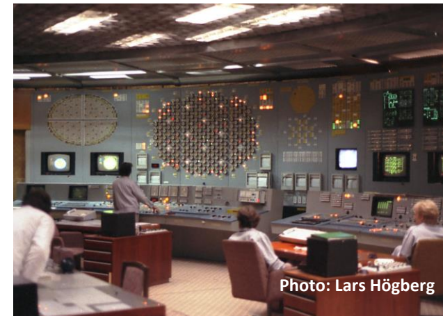
An RBMK control room (Ignalina 1990)
